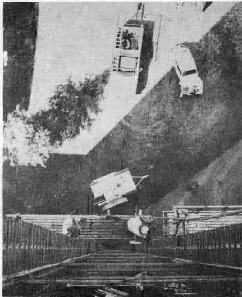
HANGIN' AROUND: Construction workers caulk cracks on the north face of the SSB tower, suspended some eight floors above the ground. The repairs were made necessary by water damage to the building [photo by Earl Swift].
